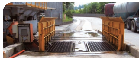
Tire washer facility
