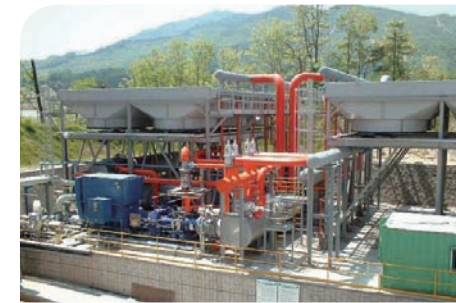
Waste heat power plant
